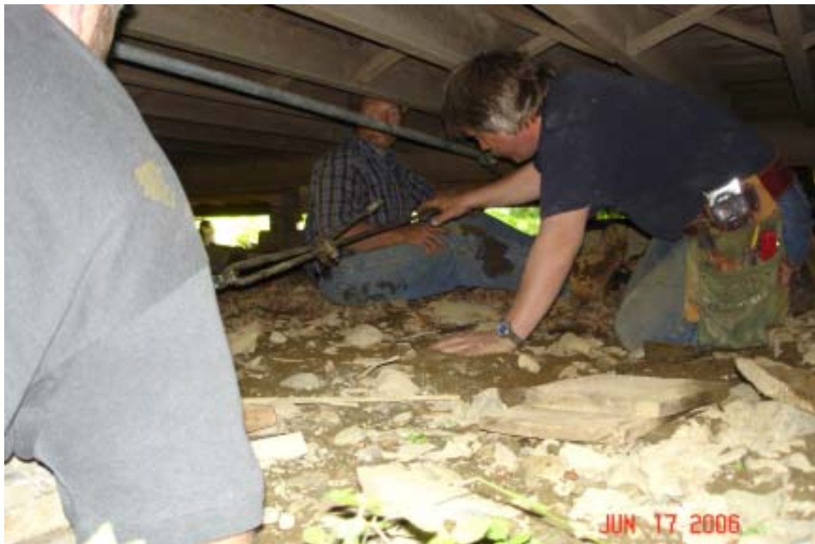
Mayo Cookson and Kenneth Overlock position the rods and cable under the hall while Clyde Rolerson passes them tools
