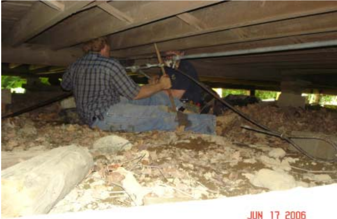
Mayo and Ken tighten the turnbuckle to pull the sides of the hall inward and the center timber upward.
